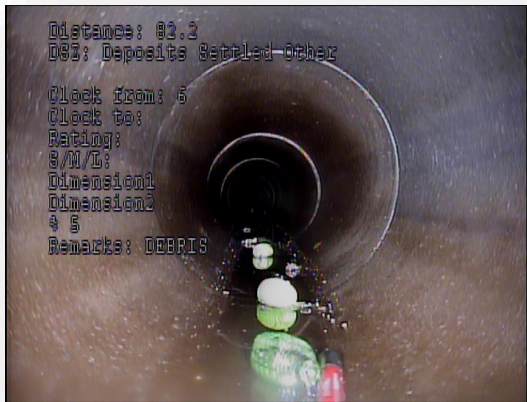
Undersized drain line between Toulouse and St. Peter streets.
