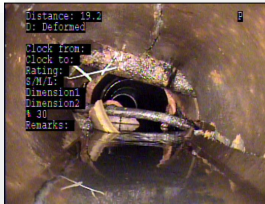
Crushed and deformed drain line between Conti and St. Louis streets.
