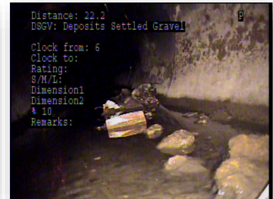
Fragments of a broken and undersized drain line between Iberville and Bienville streets.
