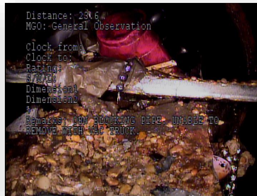
Debris filled, broken drain line between Orleans Ave. and St. Ann St.
