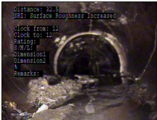
Cracked and damaged drain line between Canal and Iberville streets.
