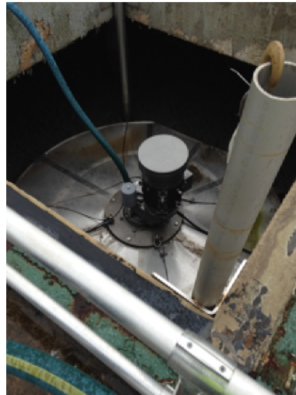
New Mixer on Reactor 1
