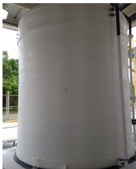
New Sodium Hypochlorite Storage Tank
