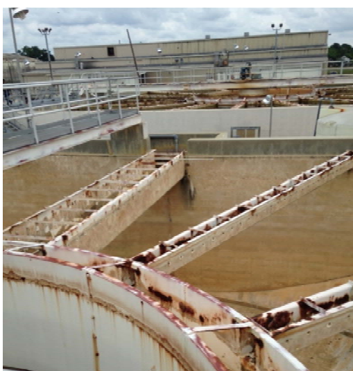
Corrosion on Clarifier Troughs
