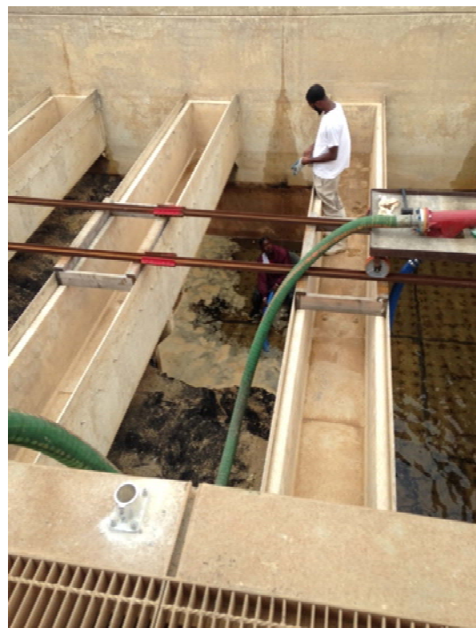
Filter Media replacement at Filter 7
