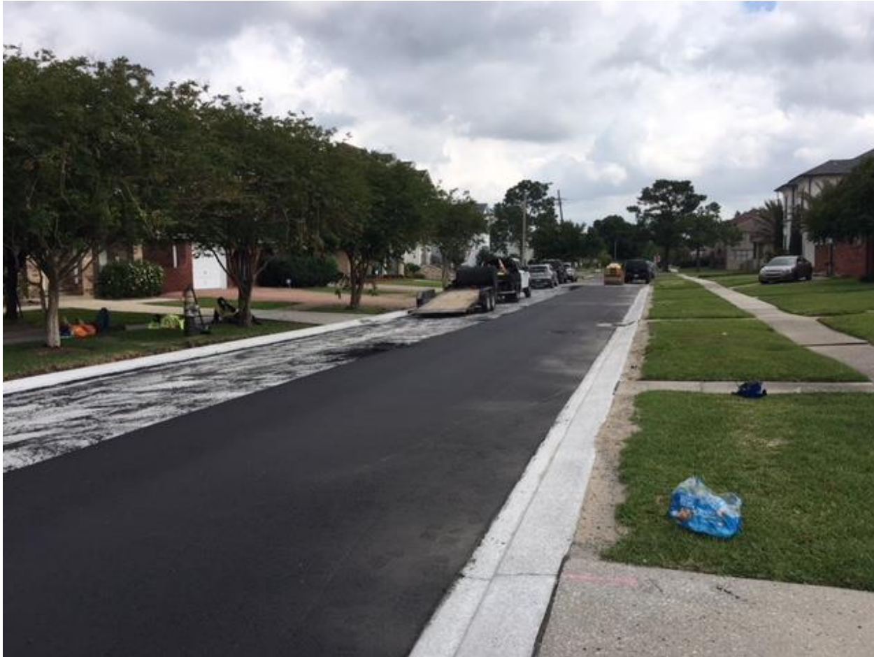
Repaving on Marshall Foch as part of the Lakeview North Group A Project
