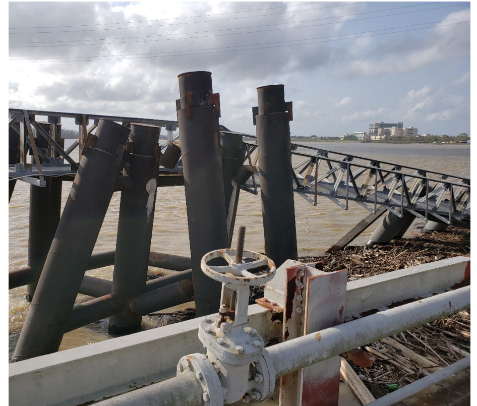
Picture of damaged Intake Fender System
