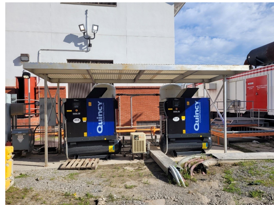
New air compressors recently installed to improve EMD reliability
