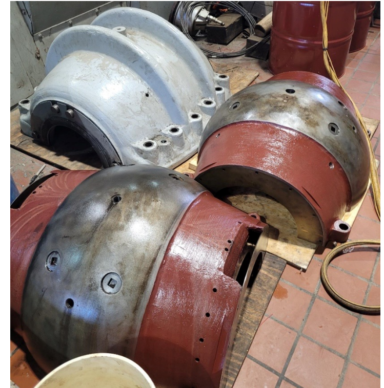
Turbine 4 bearing housing
