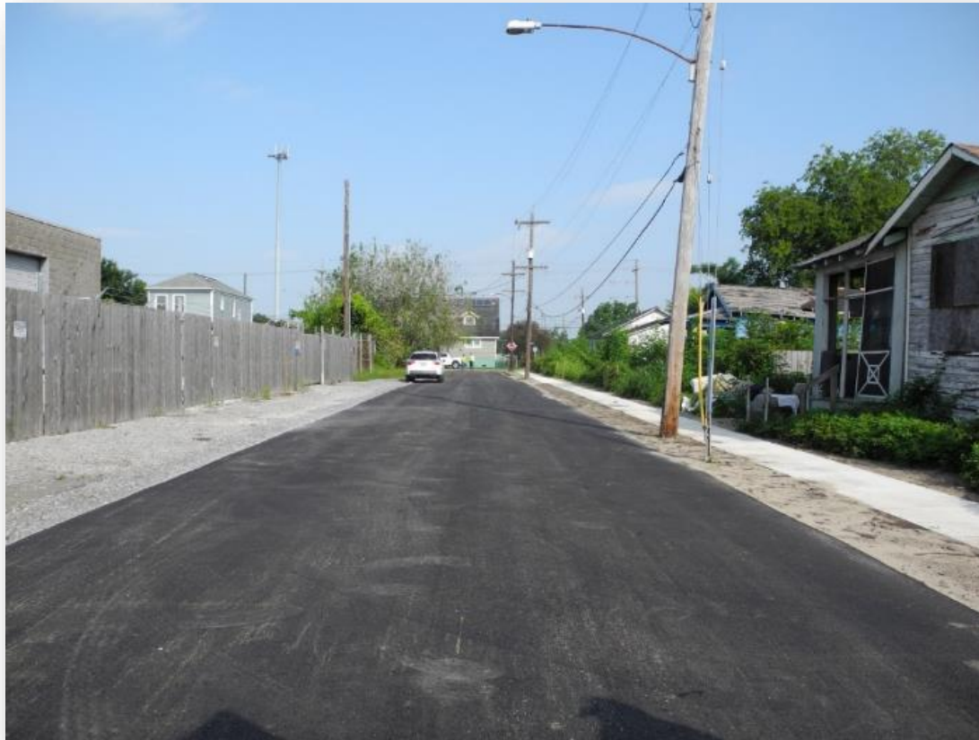
An example of a repaved asphalt road in one of our JIRR roadway projects
