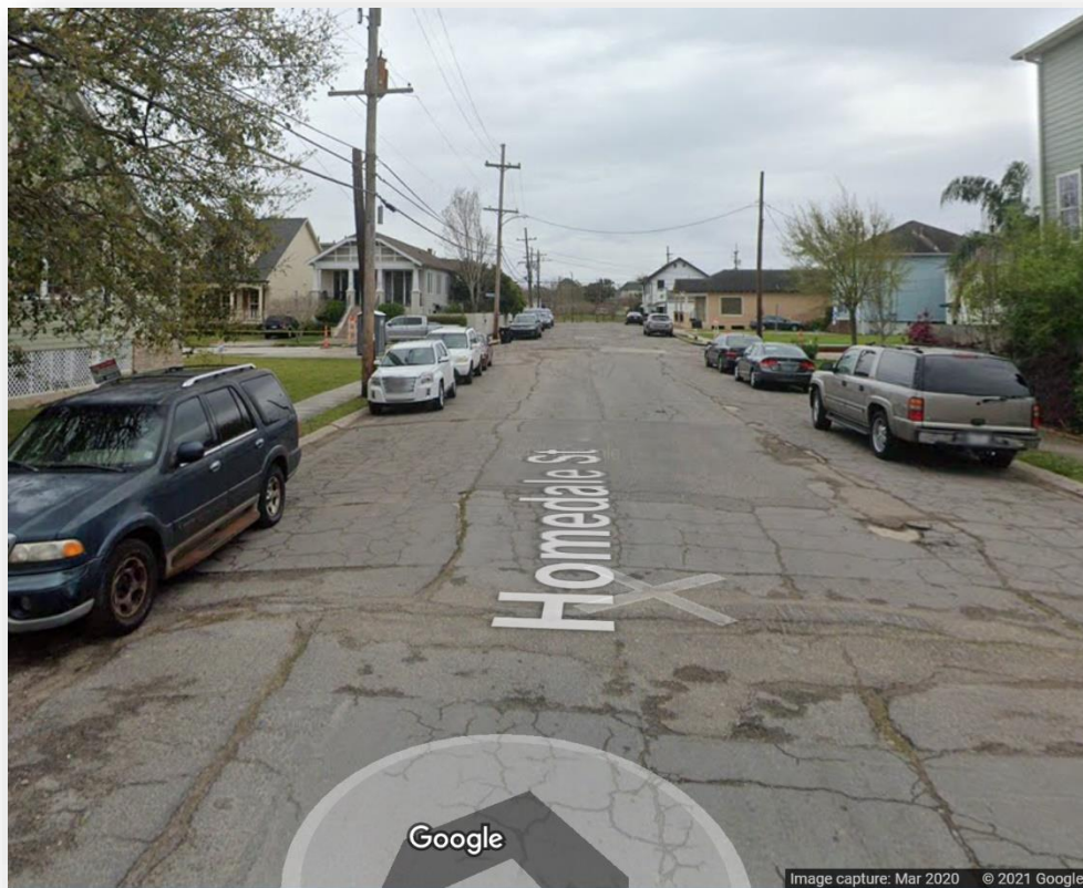
Existing asphalt conditions on the 500 block of Homedale Street
