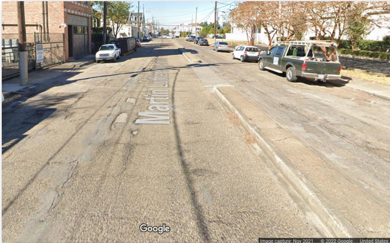
Existing asphalt conditions on the 1600 block of Martin Luther King Jr. Boulevard
